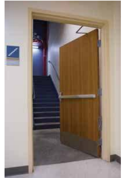
The stairwell reentry requirements vary between the IBC and NFPA 101; the IBC requires all stair doors to allow reentry with the exception of the discharge door.
