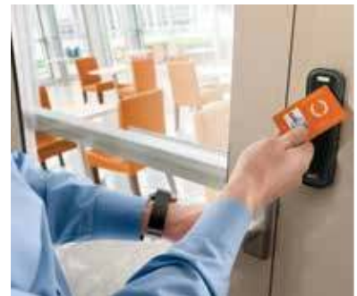
When a door equipped with an access control reader allows free egress using normal operation of the hardware, it is not typically considered one of the special locking arrangements.
