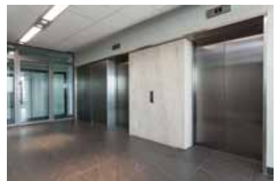
Electrified locking of elevator lobby doors is only addressed by NFPA 101, not the IBC, although some jurisdictions have adopted code modifications that allow it.
